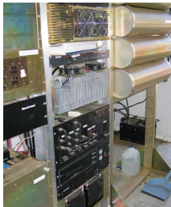
Paging base station with Zetron Model 66 Transmitter Controller.
